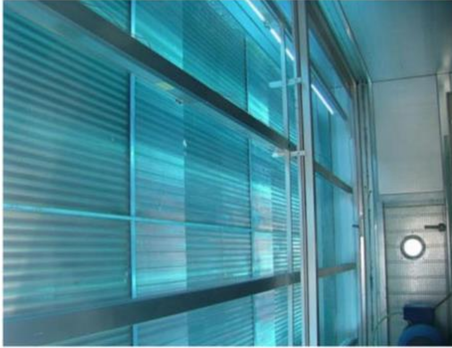
Figure 2: UV Irradiation Lamps of an HVAC System. Credit: Leach, T.; Scheir, R.; Ultraviolet Germicidal Irradiation (UVGI) in Hospital HVAC Decreases Ventilator Associated Pneumonia. ASHRAE 2014 .
